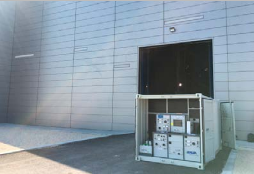
Container in front of the cable hall
