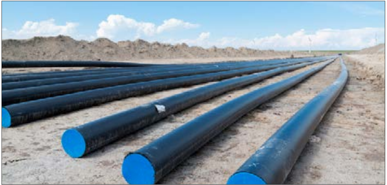
Conduits for high-voltage cables for onshore wind turbines
