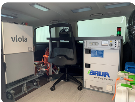
BAUR has installed everything required for cable testing, and diagnostics on medium voltage cables, for SIG in an electric van.
