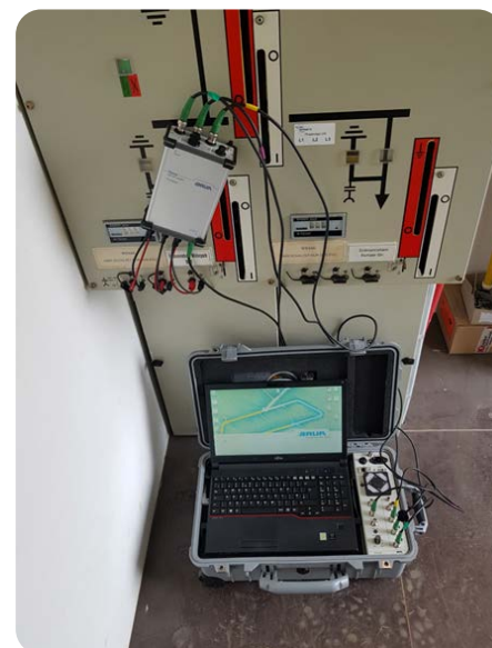
Connect whilst energised, measure while energised: The new VDS-C can identify partial discharges on cables quickly and easily during operation.
