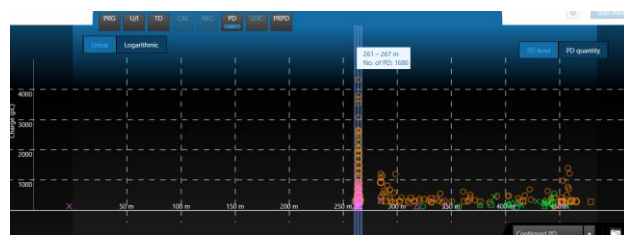
Figure 6 PD localization graph with PD in a transition joint, PD in PILC cable
