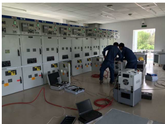
Figure 5: Field test condition, substation
