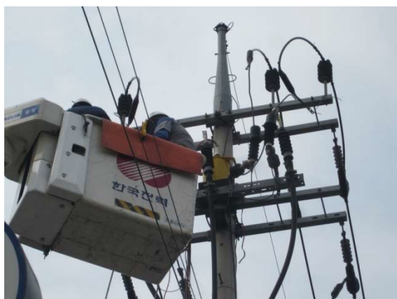
Figure 6: Field test condition, pole mounted termination
