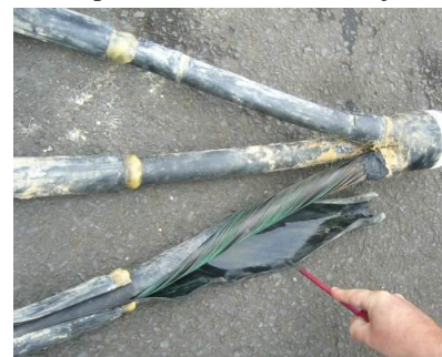
Figure 5: Joint dissection, water ingress in L3
