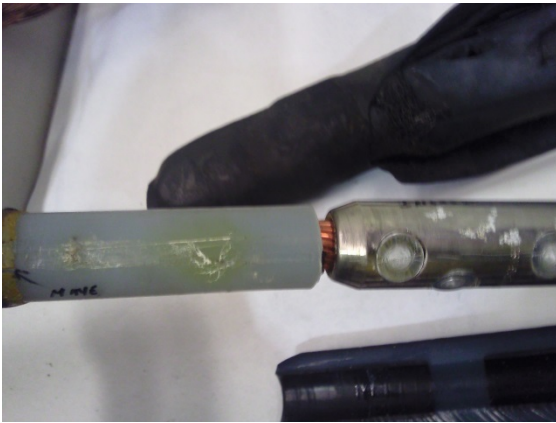
Figure 9 Joint dissection of cable #1, L1 at 350m, PD tracking mark
