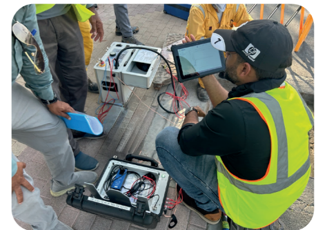
Exact fault location thanks to Step TDR
